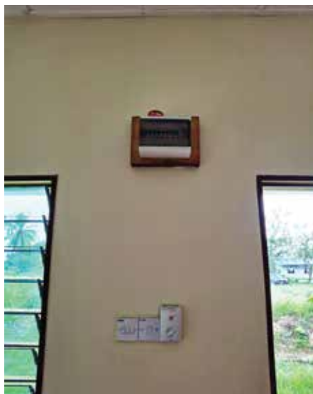
Wall switch and DB box on PRIMA Board
