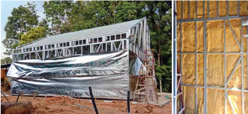
Sisalation sheets on LGS frames before install PRIMA fibre cement boards Wall insulation (optional)
