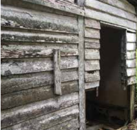
Timber is highly susceptible to rotting and termite attack
