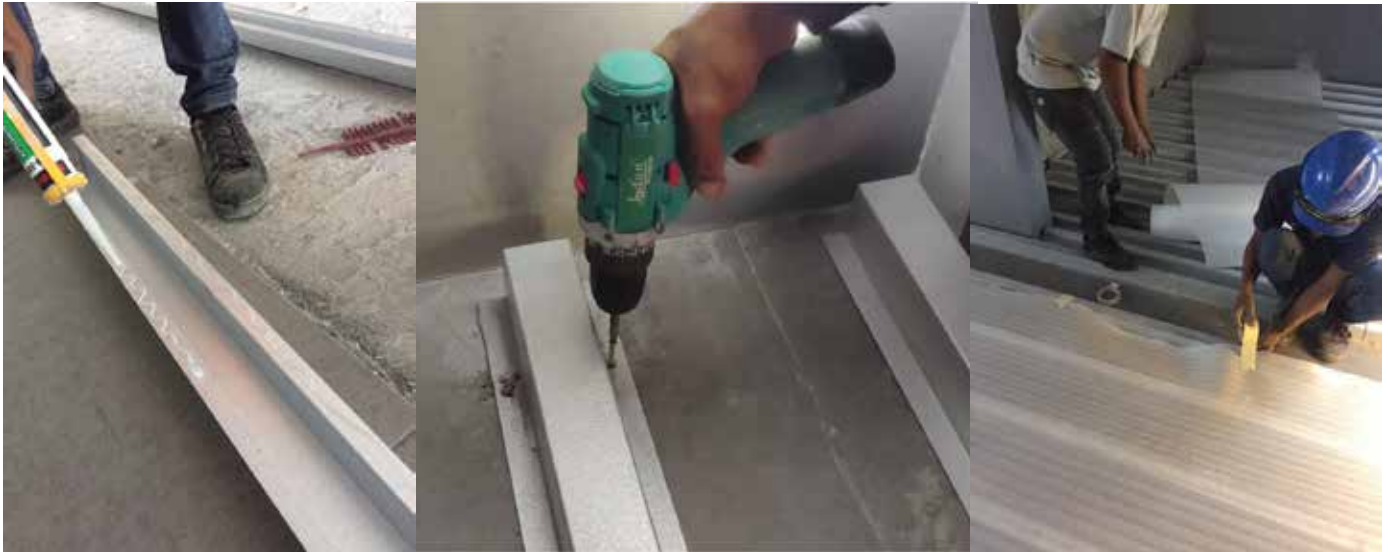
Figure 1 : Place the PRIMA Tophat 50mm x 50mm x 0.75mm BMT at the marked position and secure the frame. Lay a layer of polystyrene sheet as sound insulator on top of the frames.
