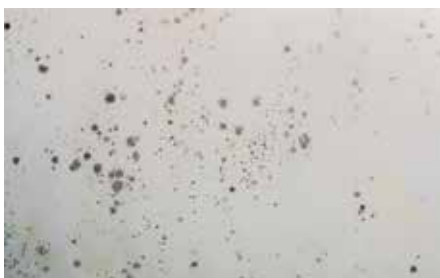
Condensation creates damp conditions causing black moulds on the wall
